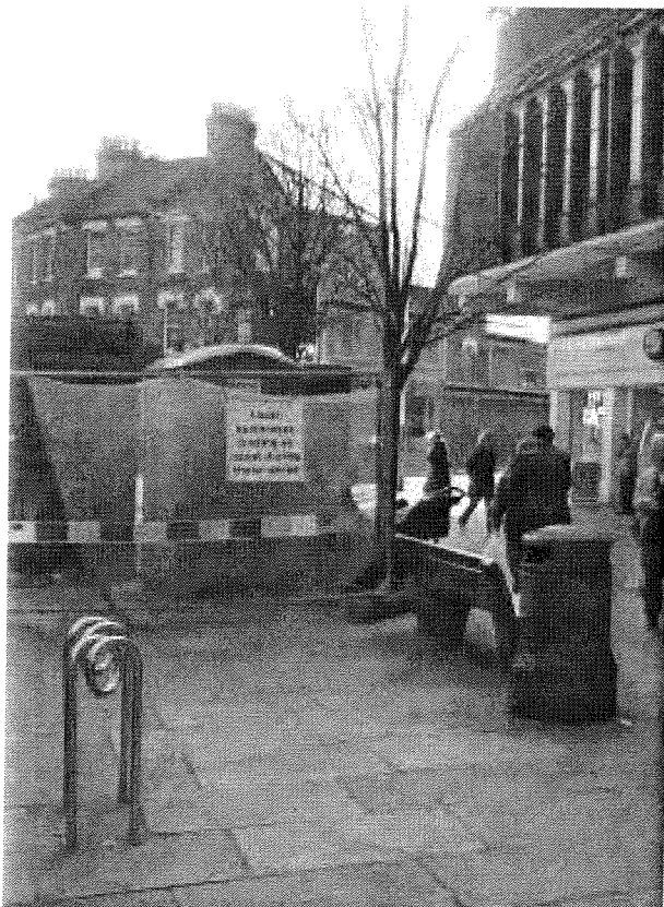
High Road - pavement obstructions
